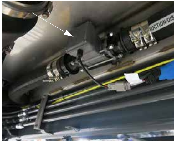
Flow Meter -Typical View
