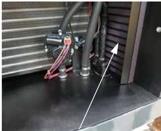
Recirculation Filter (Located along the right-hand side of service compartment) -Typical View
