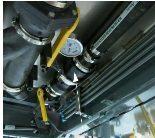
Flow Meter -Typical View
