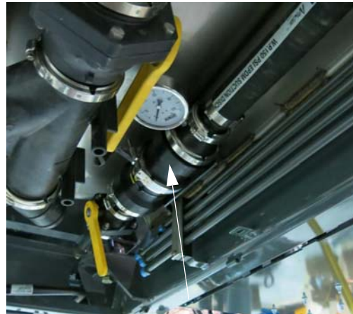
Flow Meter -Typical View
