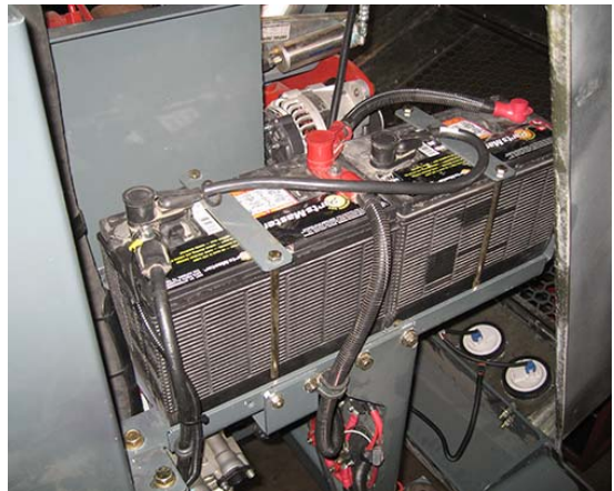
Battery Access (Located on the rear left-hand side of machine - open hood to access) -Typical View
