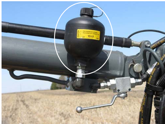
Accumulator -Typical View
