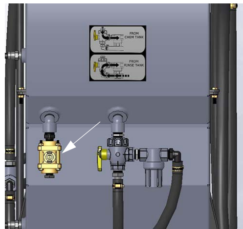
Tank Drain Valve -Typical View
