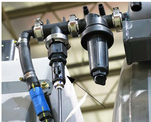
Foam Marker Valve (Located near rear of rinse tank) -Typical View
