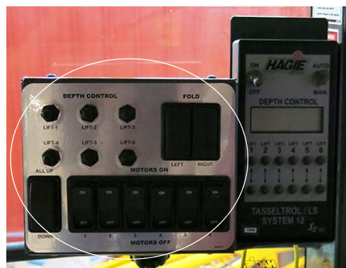
Detasseling Control Panel -Typical View
