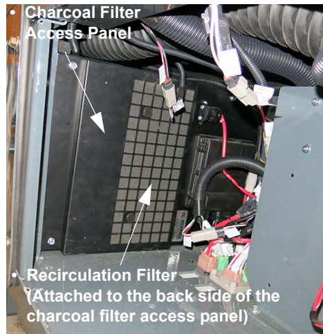
Charcoal Filter Access Panel (Located behind exterior service panel on right-hand side of cab) -Typical View
