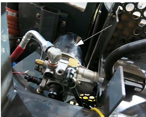
Air Dryer (Located beneath the right-hand side of machine) -Typical View
