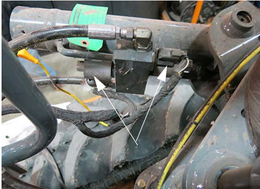
Lock Valves -Typical View
