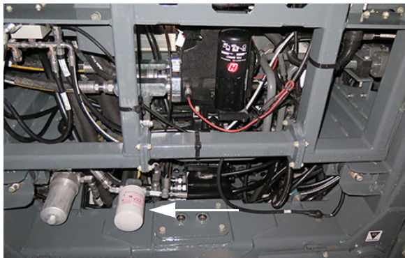
Case Drain Filter 2 (Located on left-hand side of machine ahead of engine frame) -Typical View
