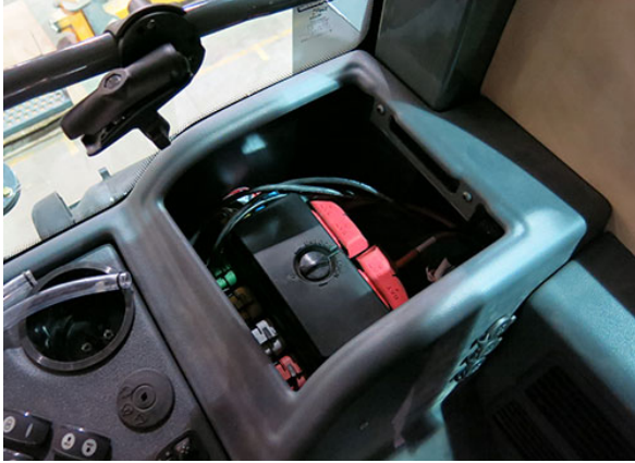
Circuit Breakers/Fuses (Interior) (Located rear of side console - remove tray to access) -Typical View
