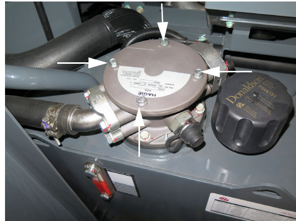
Return Filter Housing (Located on top of hydraulic oil reservoir) -Typical View
