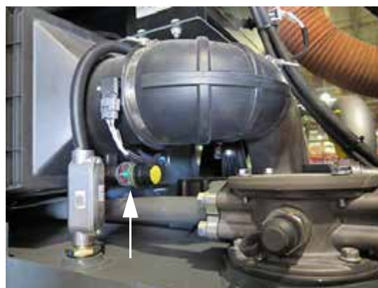
Filter Minder (Located near engine pre-filter - open hood to access) -Typical View
