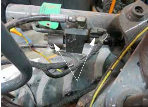
Lock Valves -Typical View
