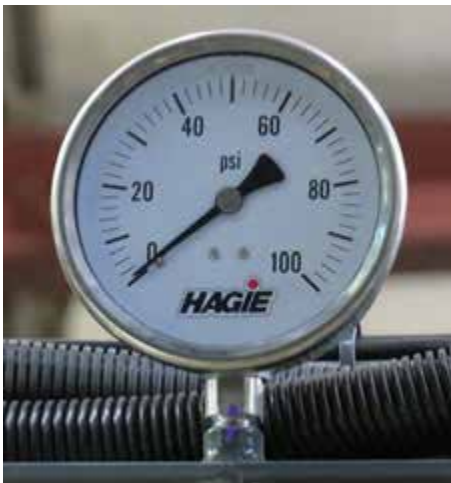
Pressure Gauge (Mounted on boom) -Typical View
