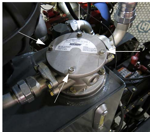
Return Filter Housing (Located on left-hand side of machine near hydraulic oil reservoir) -Typical View
