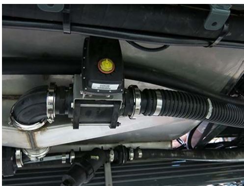
Solution Tank Valve -Typical View
