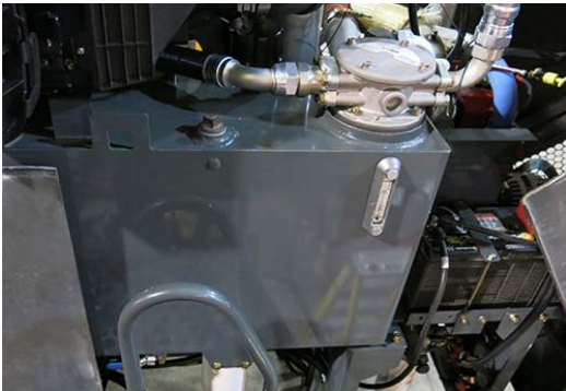
Hydraulic Oil Reservoir (Located on left-hand side of machine - open hood to access) -Typical View
