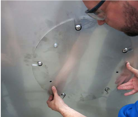
Hub Cap Access Panel -Typical View
