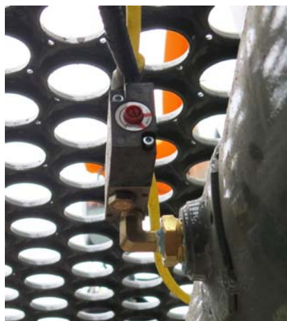
Pilot Valve (Located near air tank) -Typical View
