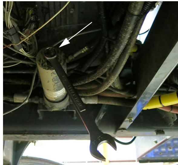
Pressure Filter Housing (Located beneath right-hand side of machine - lower metal shield to access) -Typical View
