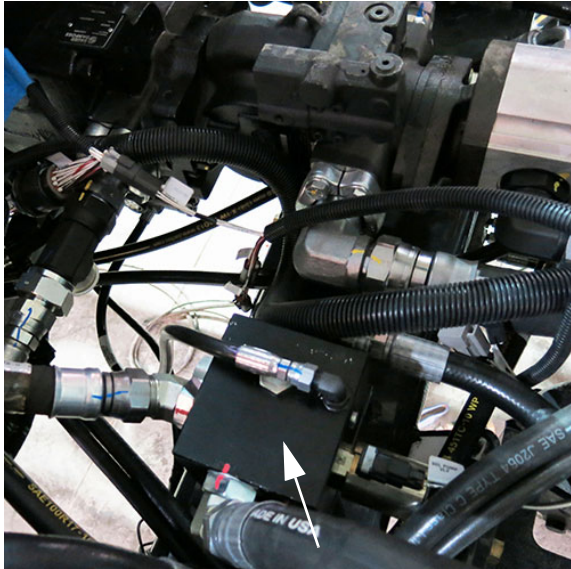
Solution Pump Control Manifold (Located near center of machine) -Typical View * View shown from top of machine
