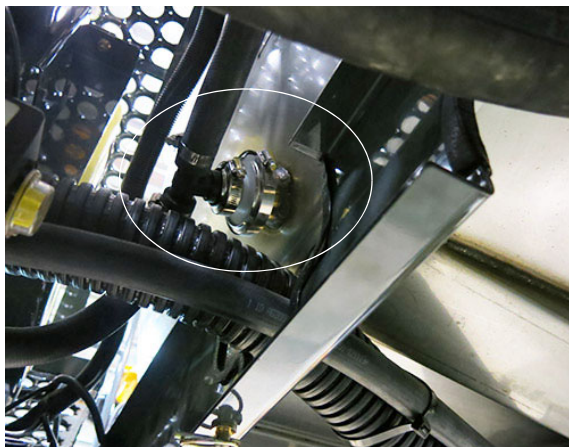
Jet Agitator (2) (Located on each end of the solution tank) -Typical View
