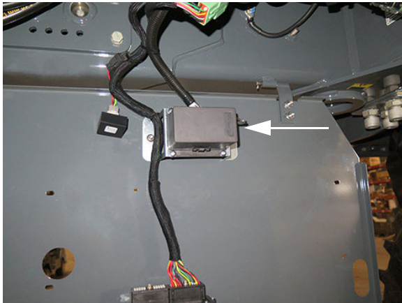
Solution Pump Relay Box (Located beneath front end of cab - lower panel to access) -Typical View
