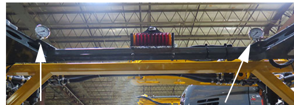
• Secondary Pressure Gauge • Primary Pressure Gauge
