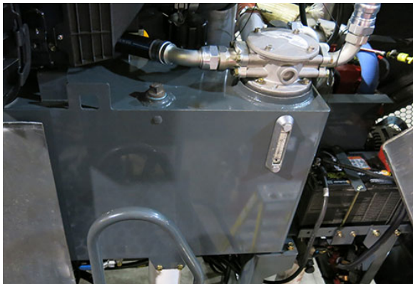
Hydraulic Oil Reservoir (Located on the rear left-hand side of machine - open hood to access) -Typical View
