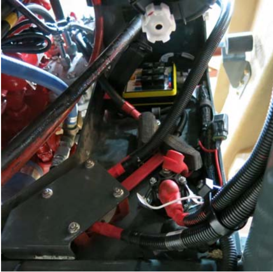
Tier 4 Final Engine Fuse/Relay Block (Located beneath batteries on the rear left-hand side of machine)
