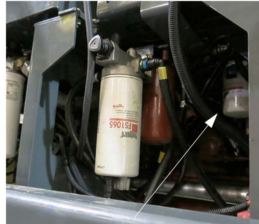
Engine Oil Filter (Located along left-hand side of machine - open hood to access) -Typical View
