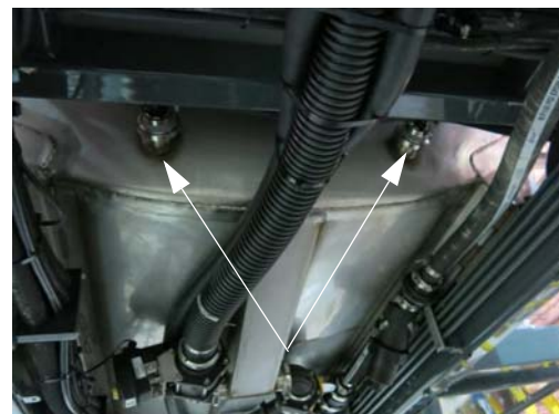
Jet Agitators (Two located on each end of solution tank) -Typical View
