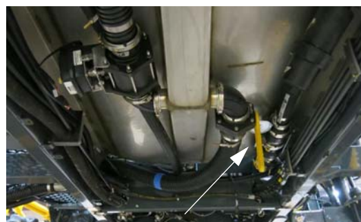
Sump Valve -Typical View
