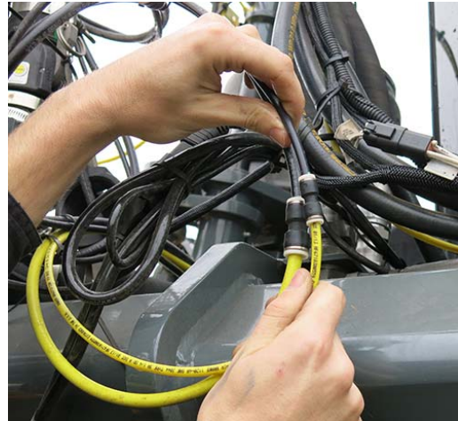
Foam Marker Connection (Located on front right-hand side of machine) -Typical View
