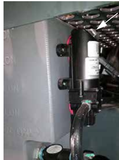
Hand Wash Pump Power Switch (Located on top of pump) -Typical View
