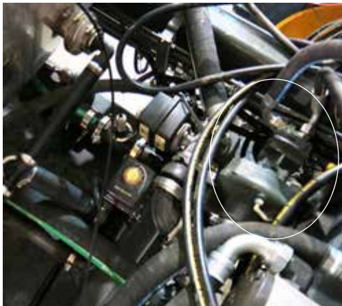
Solution Pump (Located near center of machine) -Typical View * View shown from top of machine
