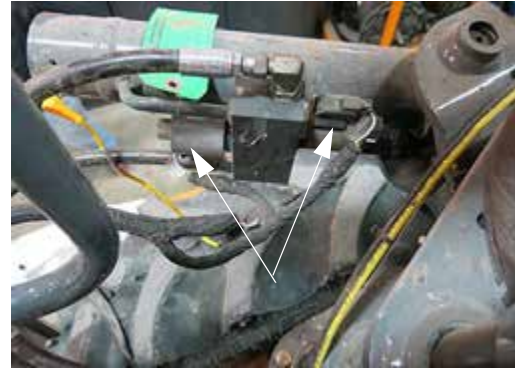
Lock Valves -Typical View
