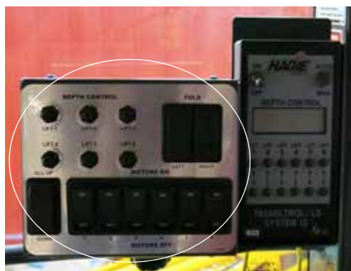
Detasseling Control Panel -Typical View
