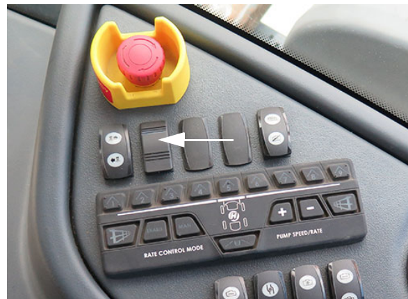
Platform Lights Switch (Located on the side console) -Typical View
