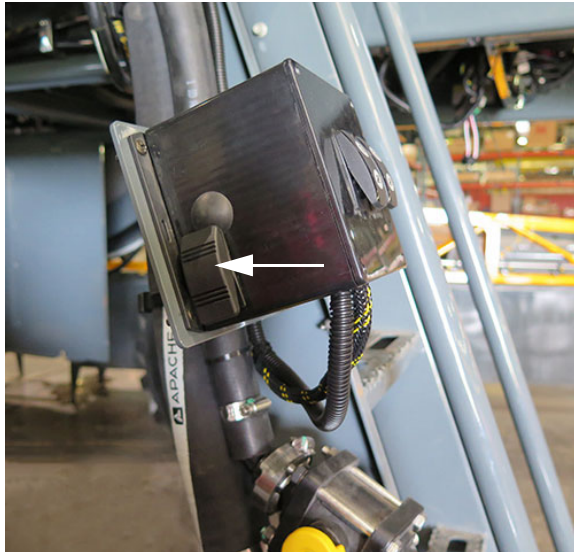
Platform Lights Switch (Located on side of switch box near ladder) -Typical View
