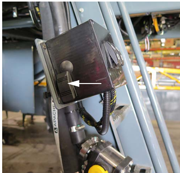
Night Spray Switch (Located on side of switch box near ladder) -Typical View
