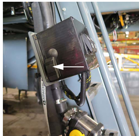
Night Spray Switch (Located on side of switch box near ladder) -Typical View
