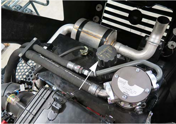
Tank Breather Cap (Located on top of hydraulic oil reservoir - open hood to access) -Typical View
