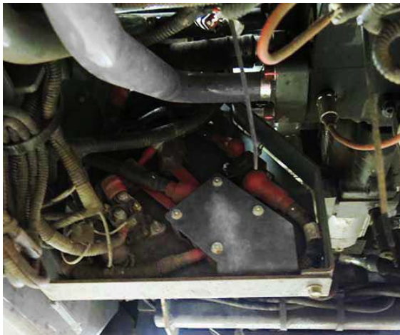
Final Tier 4 Engine Fuse/Relay Block (Located beneath batteries on the rear right-hand side of machine) -Typical View
