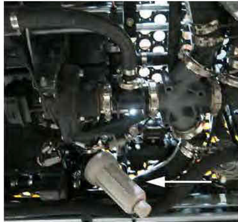
Solution Line Strainer (Located beneath center of machine) -Typical View
