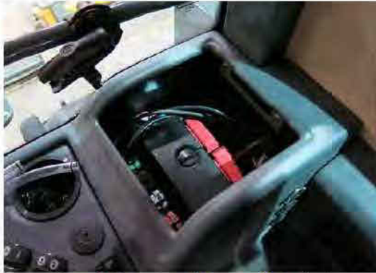
Circuit Breakers/Fuses (Interior) (Located rear of side console - remove tray to access) -Typical View
