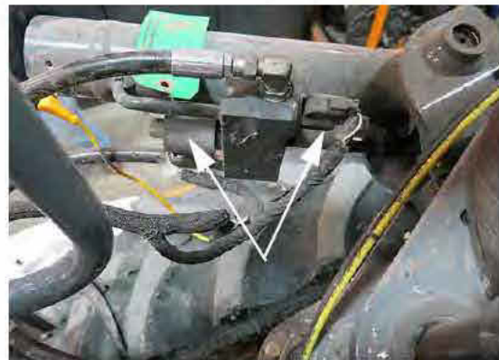
Lock Valves -Typical View
