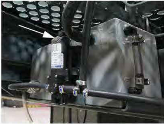
Hand Wash Pump Power Switch (Located on top of pump) -Typical View
