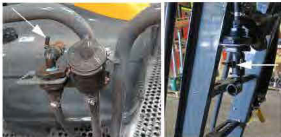
Hand Wash Valve (Left-Hand Platform Handrail)
