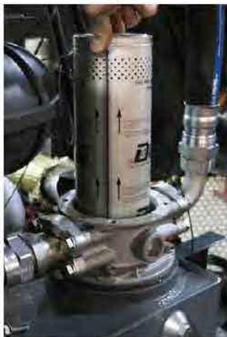
Return Filter (Located inside filter housing) -Typical View
