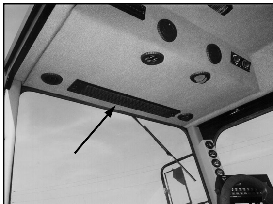
CAB FILTER LOCATION IMG 8.27
