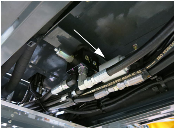
High Pressure In-Line Filter (Located beneath machine - lower front screen panel out to access) -Typical View
