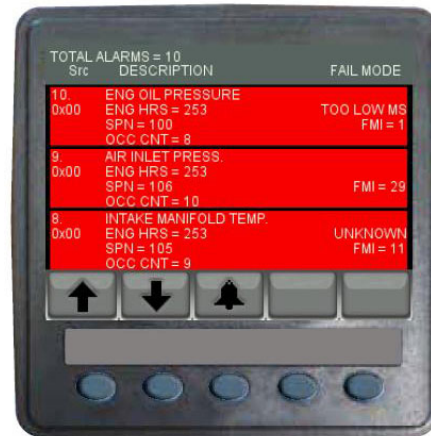
Active Alarm Screen -Typical View
