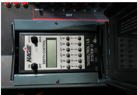
Tasselrol/LS System 12 Control Panel (Located on the side console - lift cover to access) -Typical View
