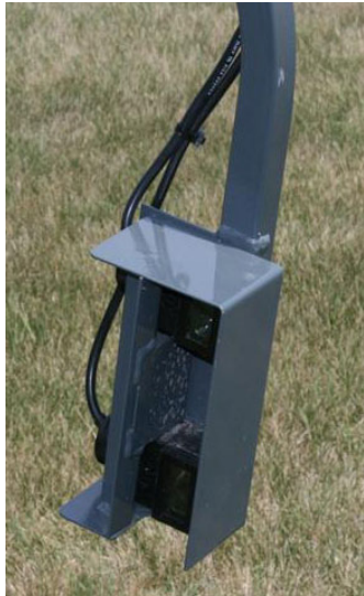
Photo Light Sensor -Typical View
