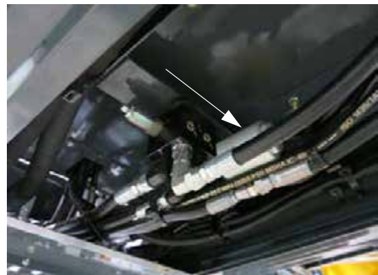
High Pressure In-Line Filter (Located beneath machine - slide screen cover out to access) -Typical View
