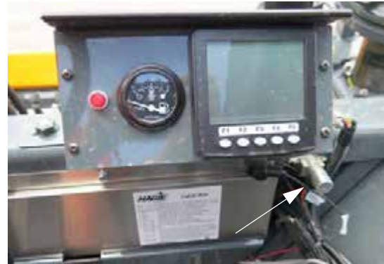
Traction Valve Switch - Front (Located near the front of operator’s station) -Typical View
