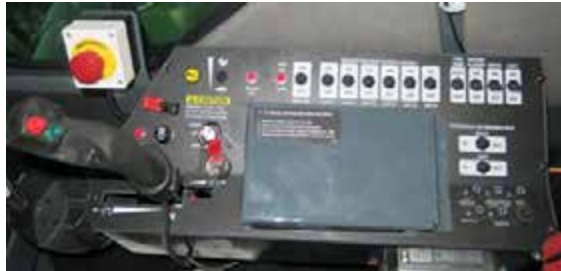
Circuit Breaker Access (Located beneath side console - remove hydrostatic drive control handle and top panel screws to access) -Typical View
