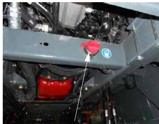
Battery Disconnect Switch (Located on the rear frame) -Typical View
